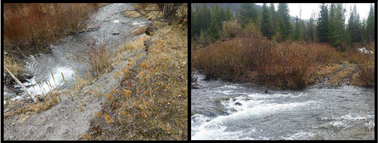
Figure 2. Photos of HACOR01 on Corbin Creek and the surrounding vegetation and nearby failing embankment.
