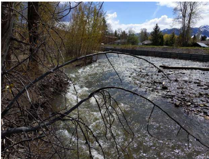
Figure 6: Rooted cut bank in adjacent to area shown in Figure 5. This bank is much more resilient to erosion, provides fish habitat, shades the water and slows water velocity during high water events.
