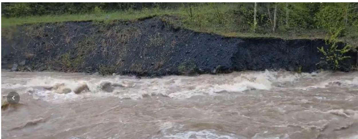
Figure 3: Same location as Figure 2 (right) during high flow event in June 2020. Note erosion at base of slope by high velocity water..
