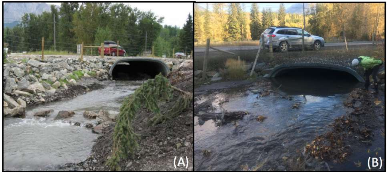
Figure 25. Comparison of the Hartley Creek culvert at Highway 3 between 2007 and 2019. (A) 2007 (photo taken by Interior Reforestation Co. Ltd.) and (B) 2019. Note compression and infilling this culvert has undergone over the 12-year period.
