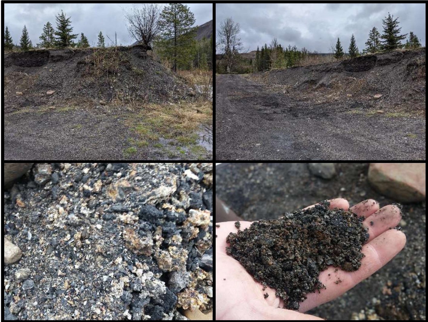
Figure 6: Failing abutment (top) and close up of abutment materials (bottom).
