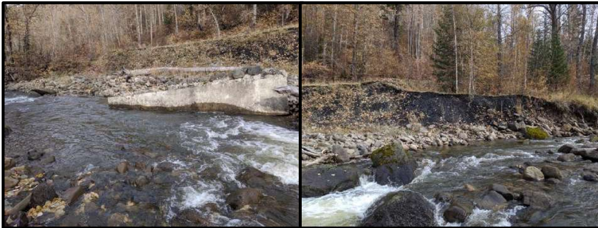
Figure 2. A historic bridge that collapsed into the stream can be seen altering the surrounding stream morphology. A failing bank can also be seen with invasive plants growing on it.
