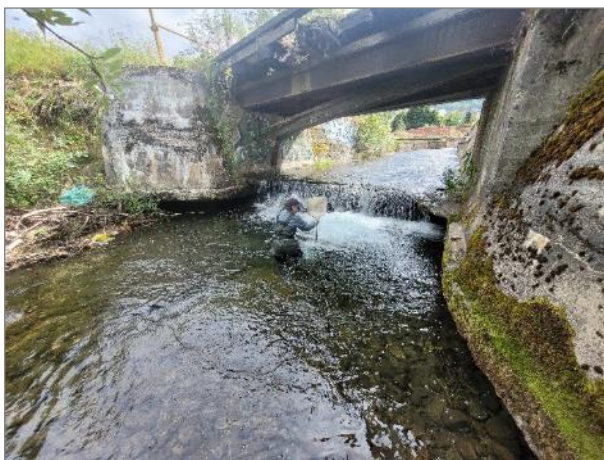
Photo 7. Plunge pool at the upstream end of R1-S2 formed at the outlet of a concrete flume.
