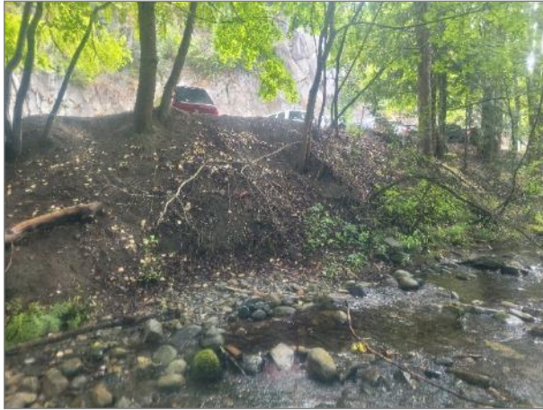
Photo 19. Section of eroded bank just below Hwy 6 Park and Ride.
