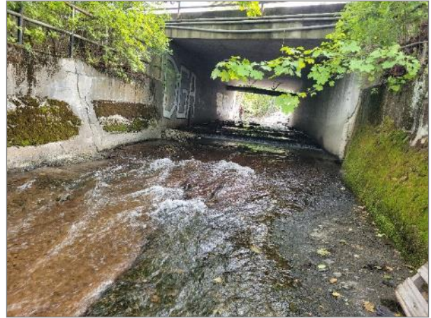
Photo 10. Representative photo of flume under Baker Street bridge, with steel baffles on bottom.
