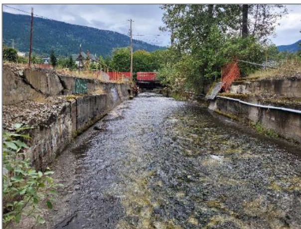
Photo 43. Concrete flume proposed to be replaced or enhanced.
