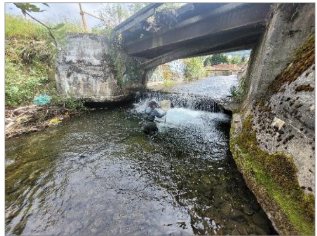
Photo 12. Obstacle to fish passage at flume outlet.
