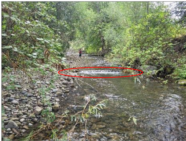
Photo 5. Representative photo of the lower portion of R1-S2, with an installed sill log. Facing upstream.
