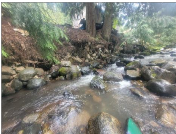
Photo 23. Section of eroded bank below a shed and driveway on residential property.
