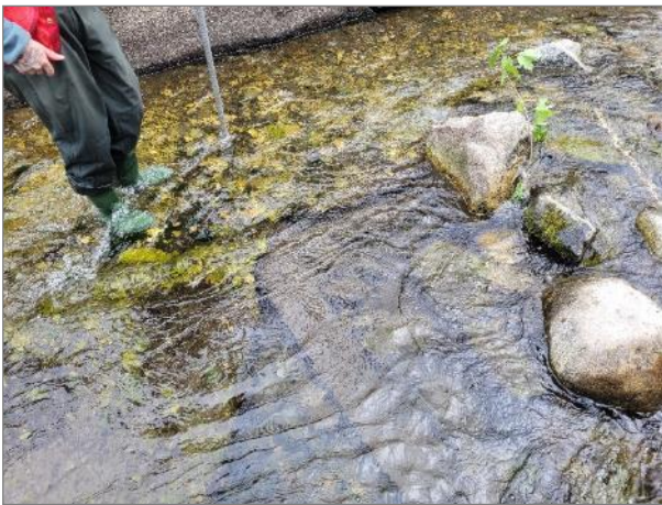
Photo 11. Example of a small pool formed where the concrete bottom of the flume had worn away.
